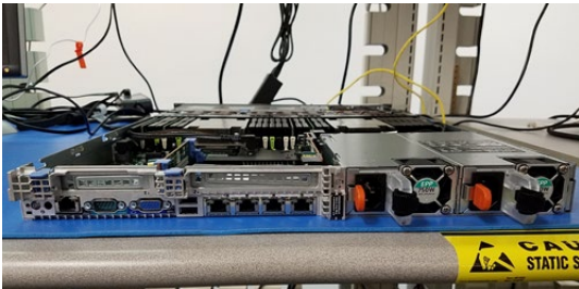
Rear server view
